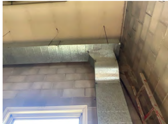
Quadville Public Works Garage - D304001
