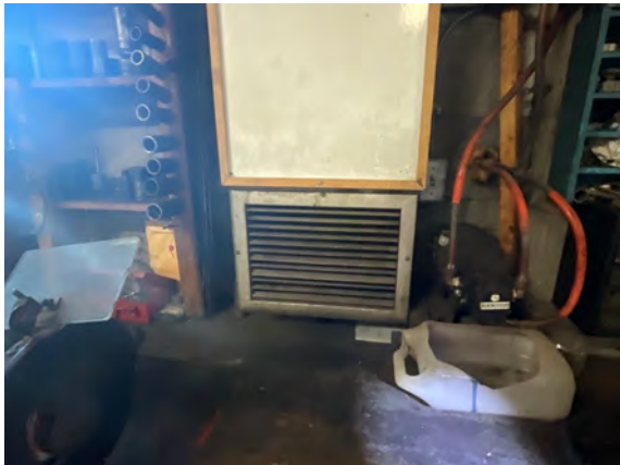
Quadville Public Works Garage - D304001
