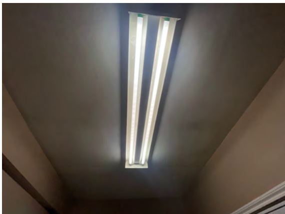
Quadville Public Works Garage - D502002
