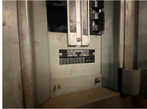
Quadville Public Works Garage - D501025
