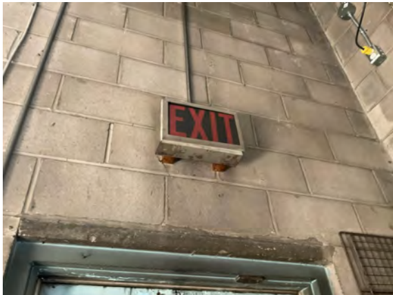
Quadville Public Works Garage - D502051
