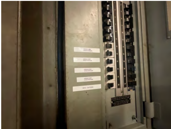
Quadville Public Works Garage - D501025
