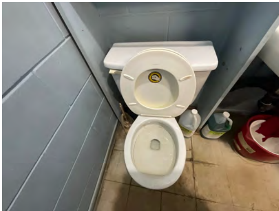
Quadville Public Works Garage - D201001
