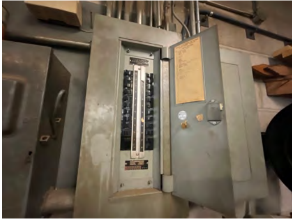
Quadville Public Works Garage - D501025
