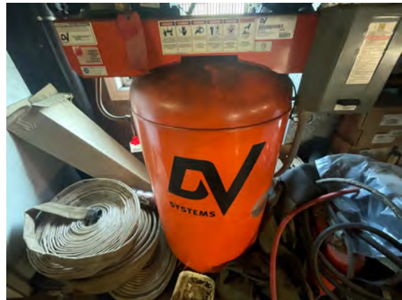
Quadville Public Works Garage - D209006
