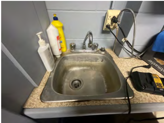
Quadville Public Works Garage - D201004
