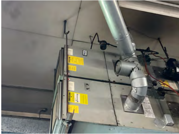
Quadville Public Works Garage - D302003
