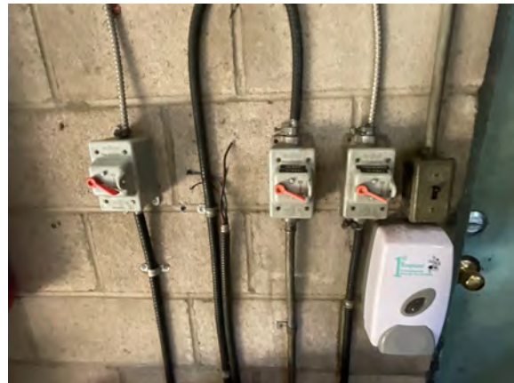
Quadville Public Works Garage - D502001
