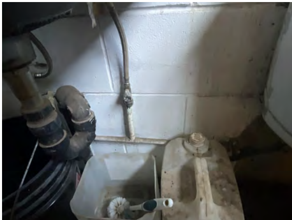
Quadville Public Works Garage - D202001
