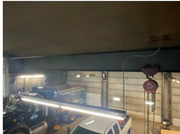
Quadville Public Works Garage - D109007
