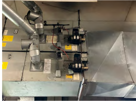
Quadville Public Works Garage - D302003
